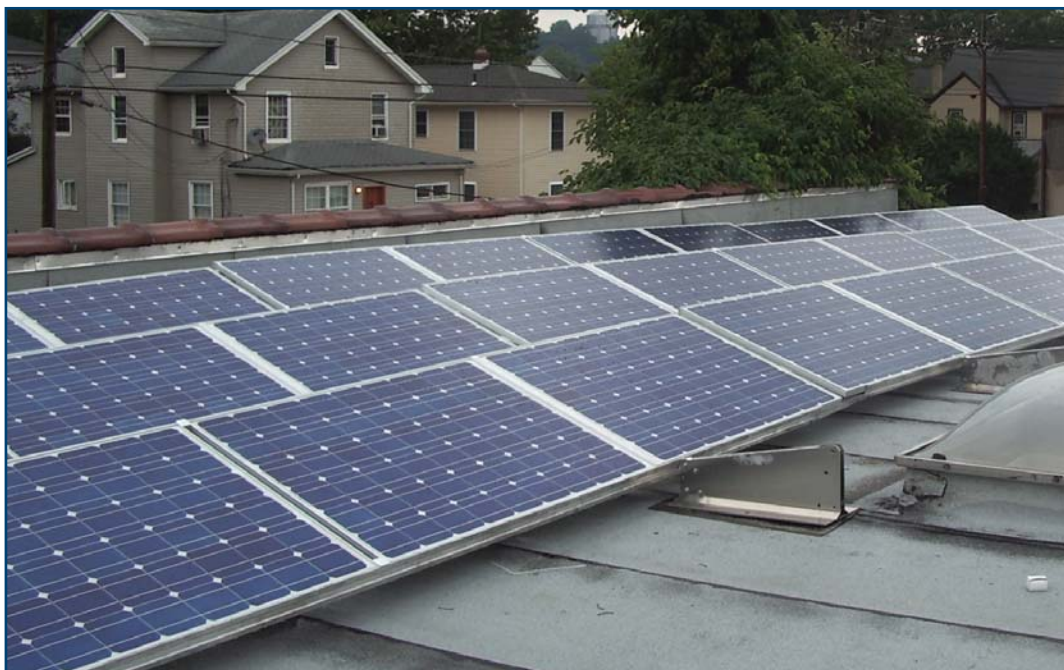
Air Systems, Kenilworth, New Jersey
