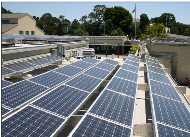
10° SunLink array at Bacich School, Marin County, CA
